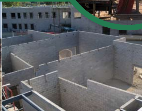
At Milkovich Middle School, classrooms are taking shape as the masonry walls go up.
