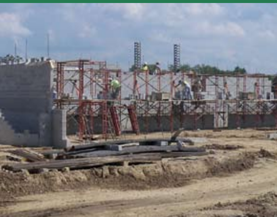
Walls are going up on the elementary campus buildings behind Dunham Elementary.
